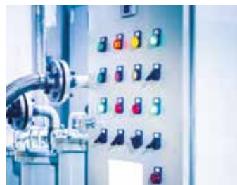
Pumping and Fan Systems
