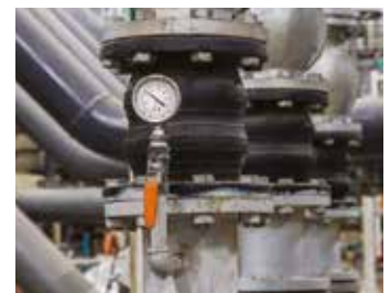
Pressurized Air Systems
