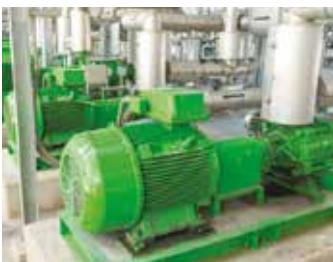
Electrical Motor Systems
